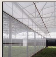
Zone Heating Curtians
